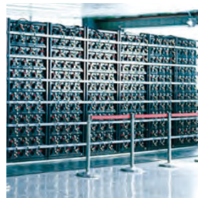
Energy storage system
