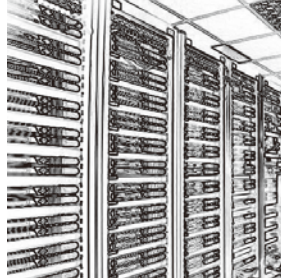
Server power supply
