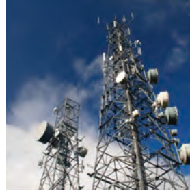
Communication power supply
